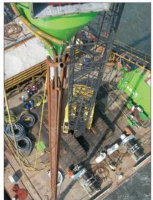
Right: View on the barge from above Rigging up the Bottom Feed Stone Column rig on a confined space of a barge requires experience. This photo was taken from the top of the auxiliary crane
