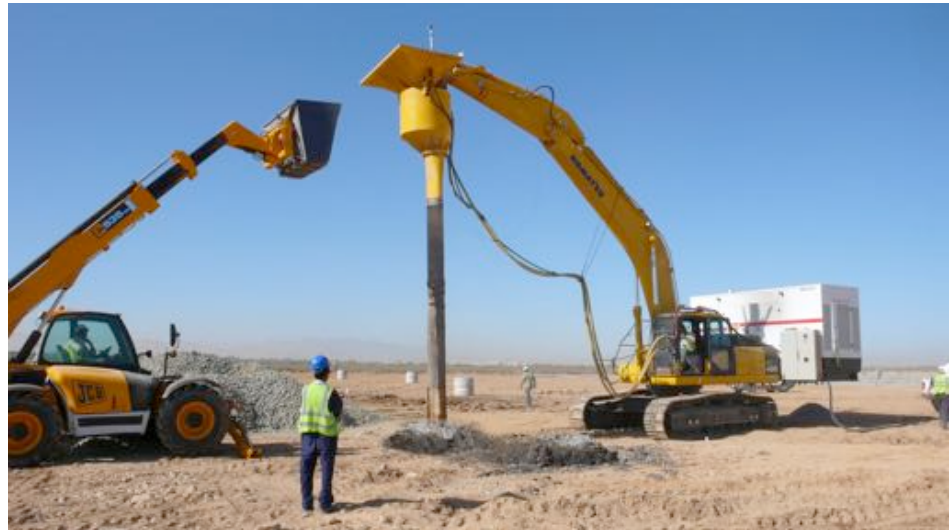
Vibro Stitcher for 6.5 m maximum treatment depth. Gravel is fed with telescopic loader.
