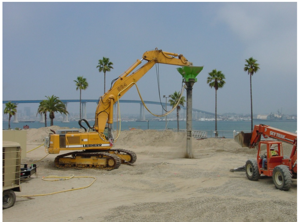
Vibro Stitcher® on a Liebherr 964 in the foreground and Cesar Chavez bridge in the background.
